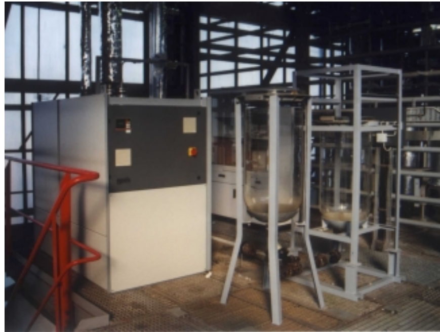
↑ platform 1: heating steam generator
